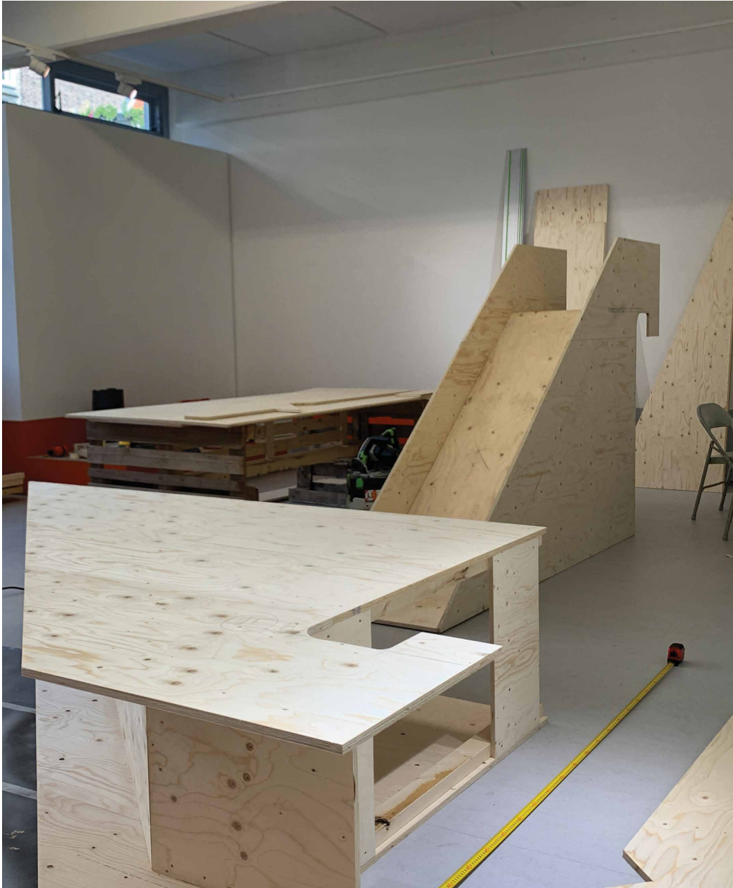
FIG. 5.14 Slides were made out of wood and varnished in the same hue as the bright green carpet. The conspicuous bright green colour was a contingent decision by the building managers based on the available affordable carpets.
