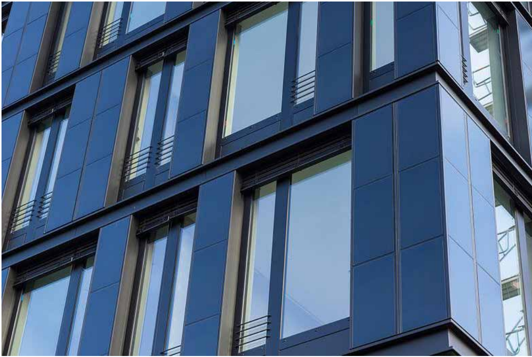
FIG. A.7 PV facade in ZSW building, Stuttgart, Germany (ZSW, 2017)
