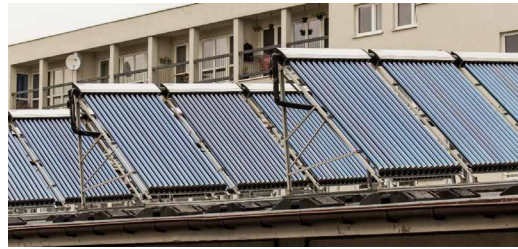
FIG. A.3 Evacuated tube collectors (Olczak et al., 2020)
