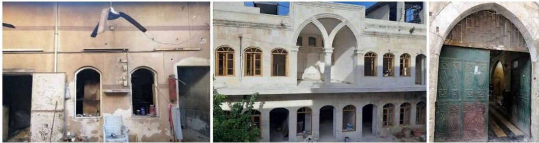
FIG. 2.5 A house that has been reused as a roastery building, Cadastral number 1479 (left), a house that has been used as a hotel, Cadastral number 1514-1515 (centre), a house that has been used as a factory Cadastral number 1427 (right), Al-Aqaba neighbourhood, Old City of Aleppo. Author and students' work, Winter 2020.
