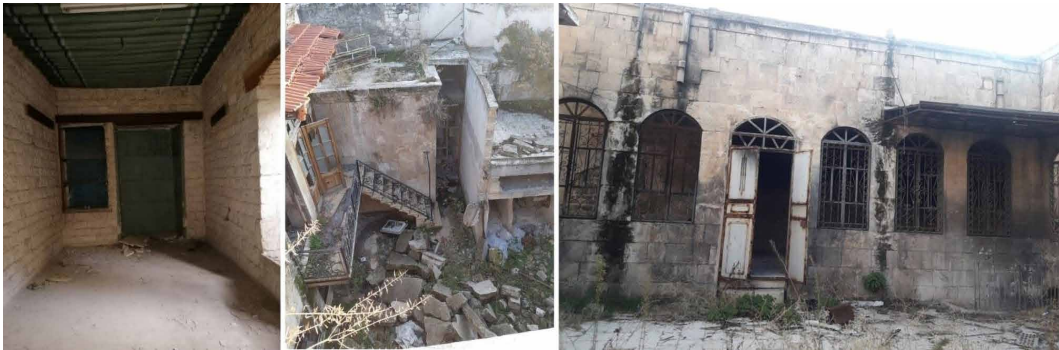
FIG. 2.6 Examples of houses that have been abandoned: Cadastral number 1453 (left), Cadastral number 1480 (centre), Cadastral number 1429 (right), Al-Aqaba neighbourhood, Old Aleppo. Author and students' work, Winter 2020.
