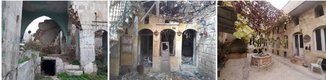
FIG. 2.3 A house that was completely destroyed, Cadastral number 558 (left), a house that was severely damaged, Cadastral number 568 (centre), a house that was not affected, Cadastral number 576 (right); Al-Jalloum neighbourhood, Old City of Aleppo. Author and students' work, Winter 2020.
