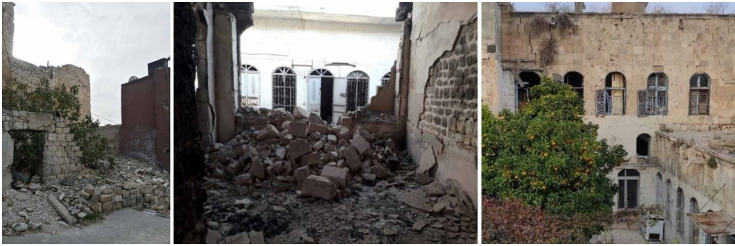
FIG. 2.4 A house that was completely destroyed, Cadastral number 1426 (left), a house that was severely damaged, Cadastral number 1429 (centre), Bullet holes from the fighting, on the façade of the house at Cadastral number 1424 (right); Al-Aqaba neighbourhood, Old City of Aleppo. Author and students' work, Winter 2020.
